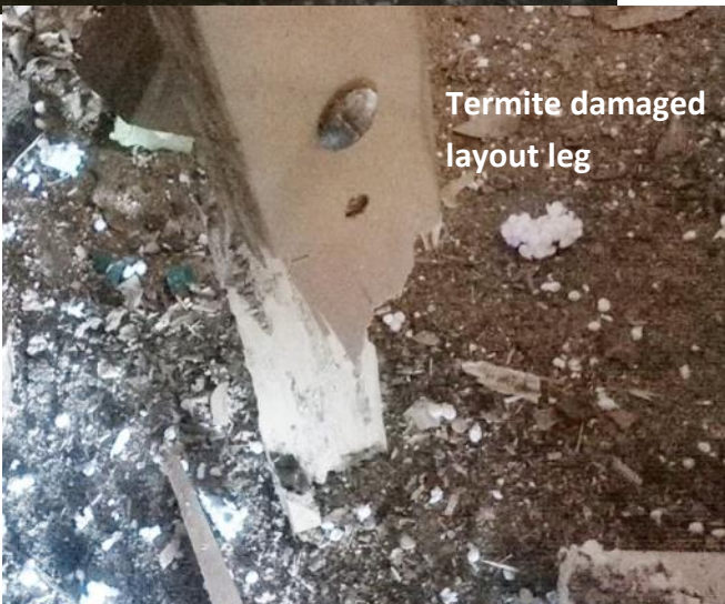
Termite damaged L girder
