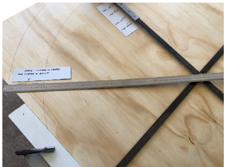
3 Mark trackbed with a ruler extending from the centre, then cut the end of section square with a Drop Saw
