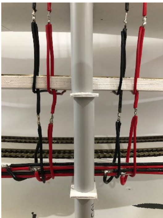
14 Connection of Track Droppers to Vertical Bus Wiring
