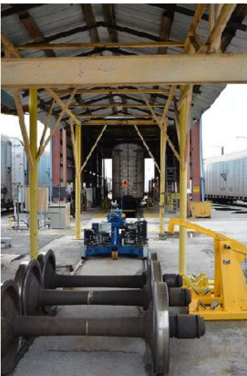
7 Pit Repair Track
