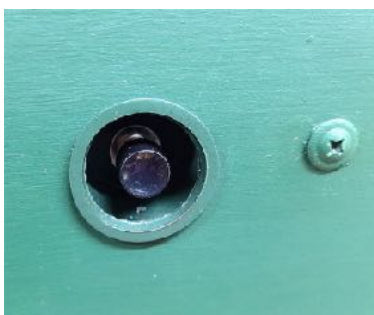
6 A Closer view of the recessed switch
