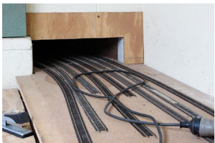
This was the entrance to the loop under the house. The eight tracks, which are in the process of being reclaimed, split into four on the other side of this wall to form the loop.
