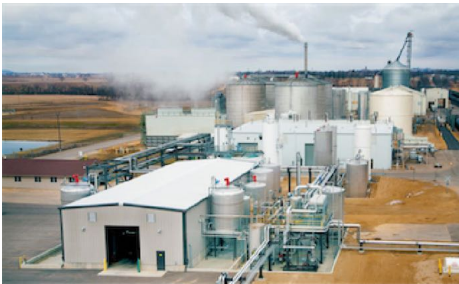
Here is one such plant I found on Google. The buildings and distribution pipes looked like they could be scratch built.
