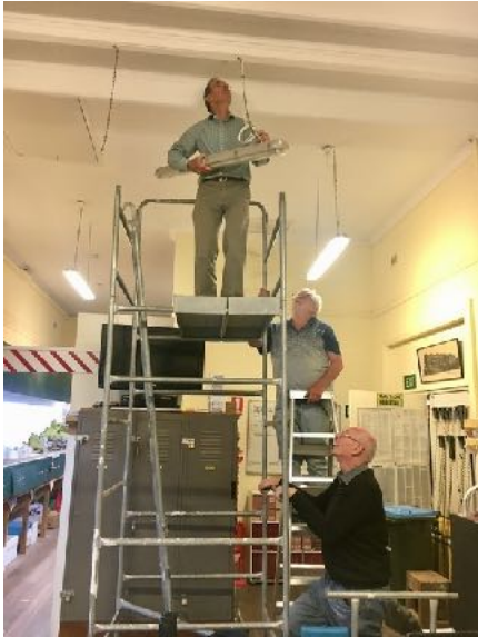
Left: Look up guys. Warwick Graham, Murray Dent and Peter Kirkland taking down one of the light fittings in the meeting area. The club has numerous LED tubes left over from changing the lighting over the layout from fluorescent tubes to LED tubes. More electricity can be saved by changing the meeting area lighting from fluorescent to LED.
