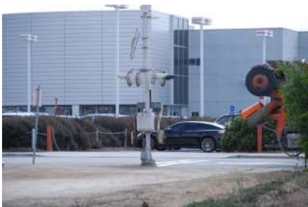
Out of service signals at Seaside CA
