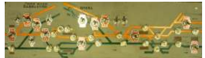
Figure 1 – Banbury Control panel which controls over 20 trains an hour through Banbury Station
